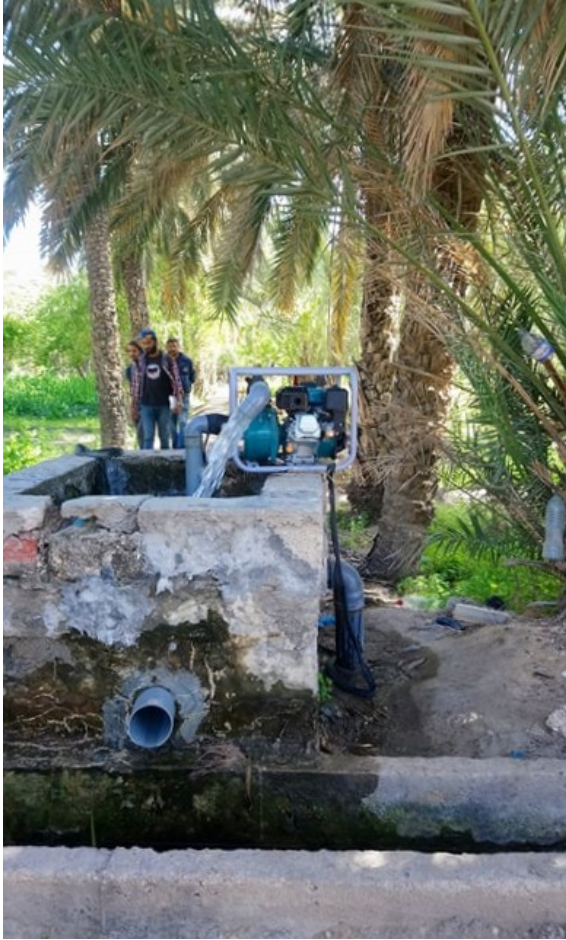
Illegally installed water pump that supplies water for the agricultural fields of five farmers in Chatt Essalam (photo: Nele Vanderpoorten)
